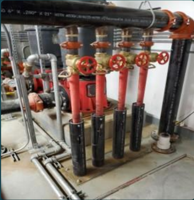
TEST HEADER RETURNING TO WATER STORAGE TANK
