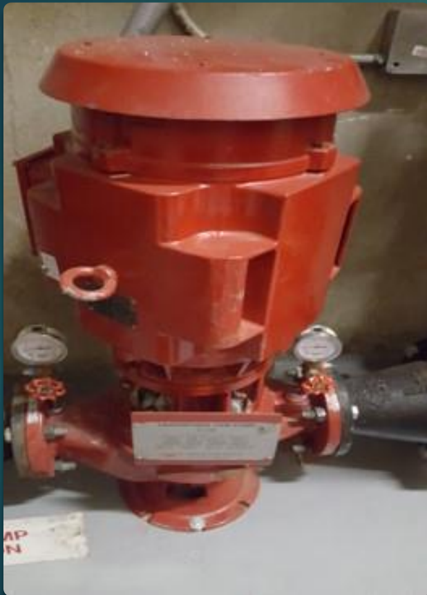
ELECTRIC INLINE FIRE PUMP
