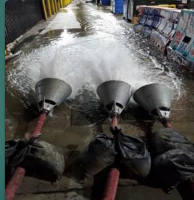
FLOW TESTING WITH PLAYPIPES AND DIFFUSERS
